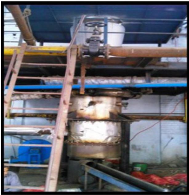
Figure 1: Downdraft gasifier (throat-less) for wood at the Chanderpur works
