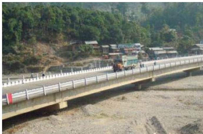
Photo 2. Sediment Accumulation under the Lothar High Bridge.
