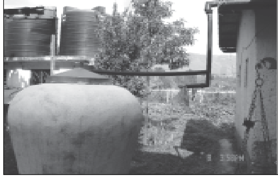
Roof water harvesting using ferro cement jar (Jhikhu Khola, Nepal)
