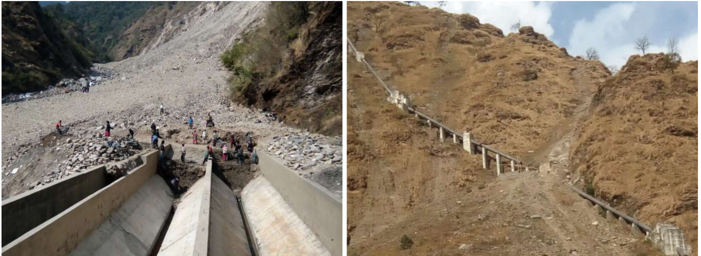
Fig. 7: Buried weir, re-excavated settling basins (Photo: Bishwo Vijaya Shrestha) and ruptured penstock pipe
