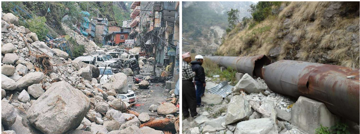
Fig. 2: Severely damaged Tatopani village (Photo: Kantipur) and ruptured penstock pipe by landslides and rock falls of the Mailung project
