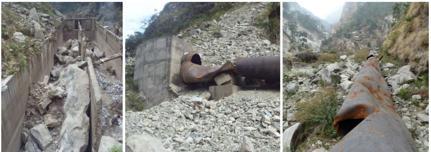
Fig. 5: Damaged settling basin and ruptured penstock pipes
