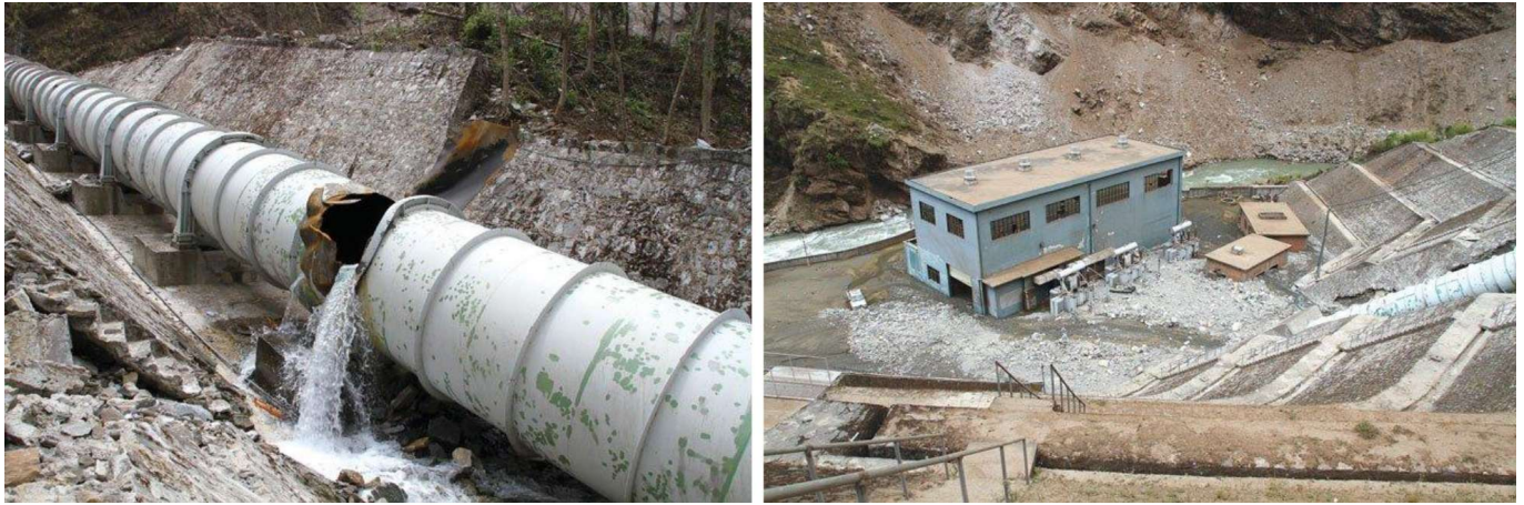
Fig. 4: Ruptured penstock pipe by rock falls and flooded powerhouse immediately downstream (Photo: Kantipur Daily)
