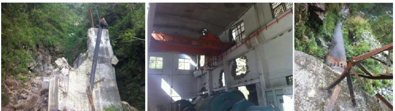
Fig. 6: Destroyed Forebay, punched powerhouse walls/roof and squeezed penstock pipe (Photo: Soyuz Gautam)
