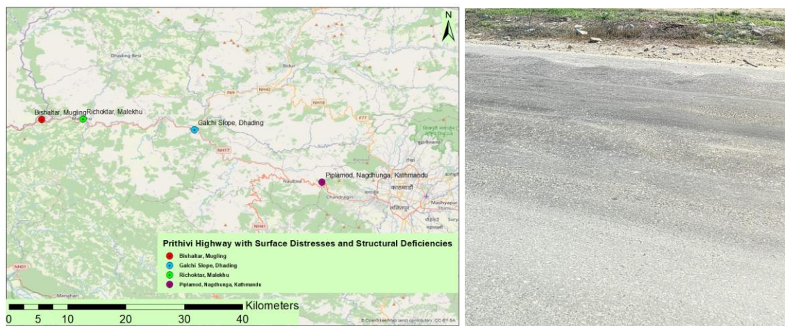
Figure 1. Surface distress and structural deficiencies identified at Bishaltar, Dhading on the Kathmandu-Mugling section of the Prithvi Highway: Location map (L-Figure), Road condition at Bishaltar (R- Figure)
