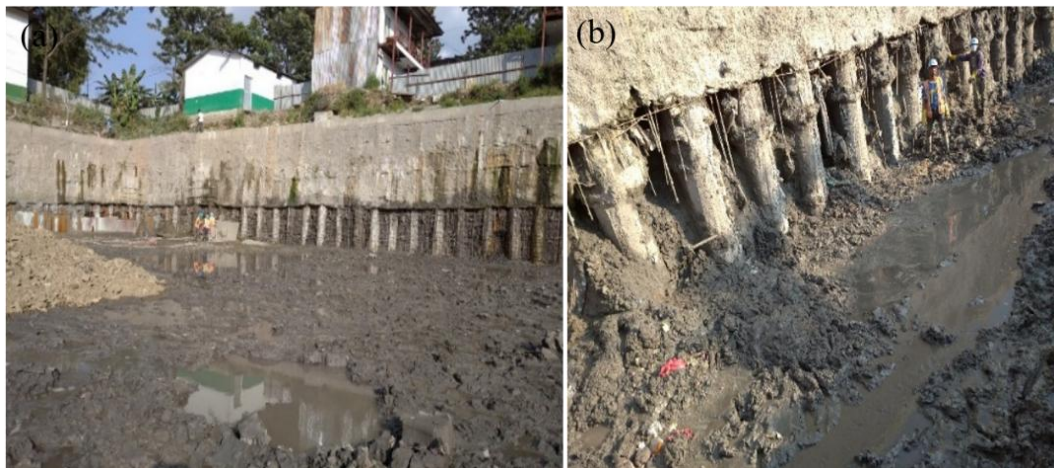
Figure 1. Study area (Ramshahpath, Kathmandu): (a) piling and jacketing construction works, (b) preparation of structural jacketing
