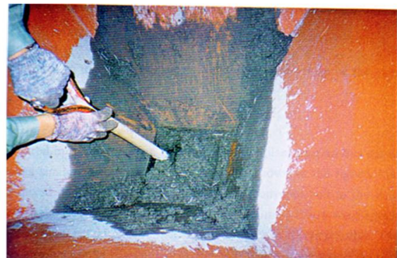
Photo 2 Condition of pre-mixed concrete and SF blocked
