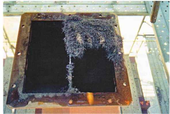
Photo 4 Condition of fiber remaining inside
