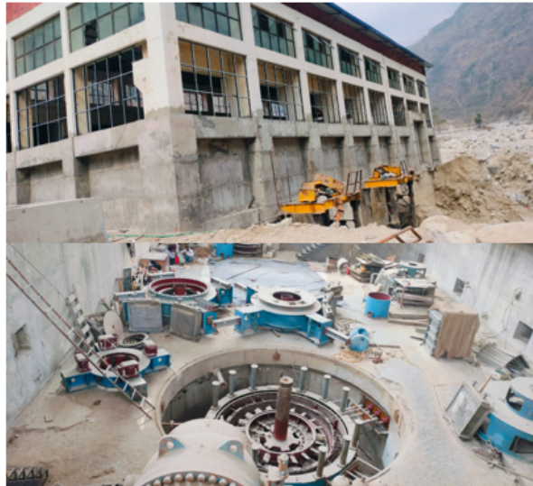
Figure 3. Damage and reconstruction of Mandu HPP
