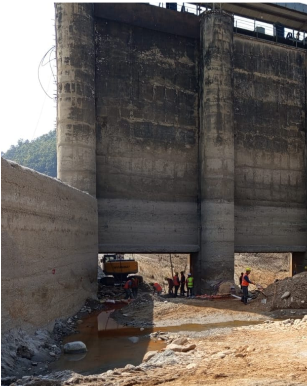
Figure 1. Damaged gate of Trishuli HPP
