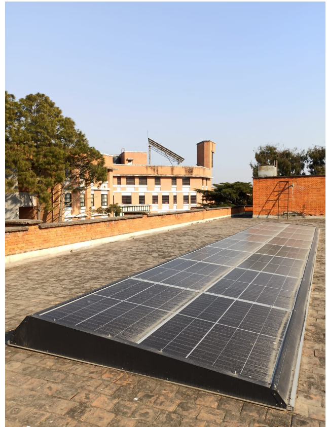
Figure 1. A 6.4 kW grid-connected PV system loaded on rooftop of Department of Electrical Engineering
