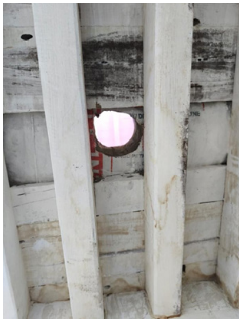
Fig. 15: Toilet basin hole of toilet no. 1 as pictured from the chamber below
